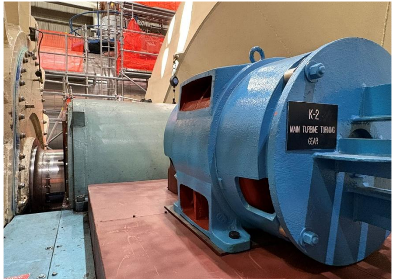
The Palisades turbine-generator on turning gear, an important step in preparing the plant's power generation equipment for operation.
