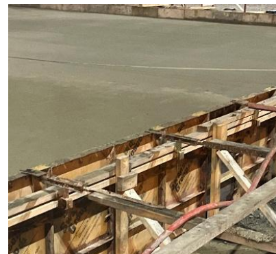
ISFSI Concrete Pad
