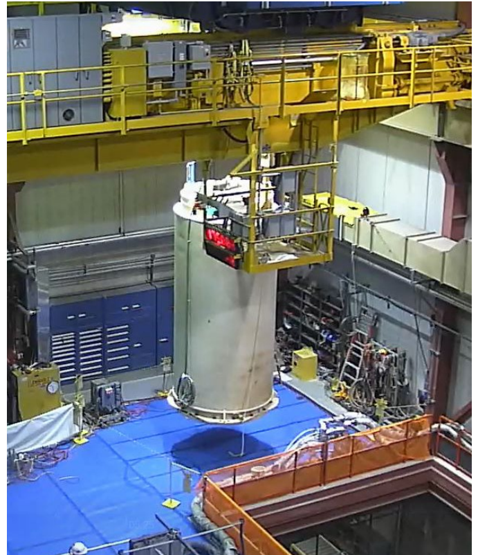
Pilgrim Crew Lifting a Multi-Purpose Canister, Which Will be Used to House Used Fuel Assemblies When Removed from the Spent Fuel Pool
