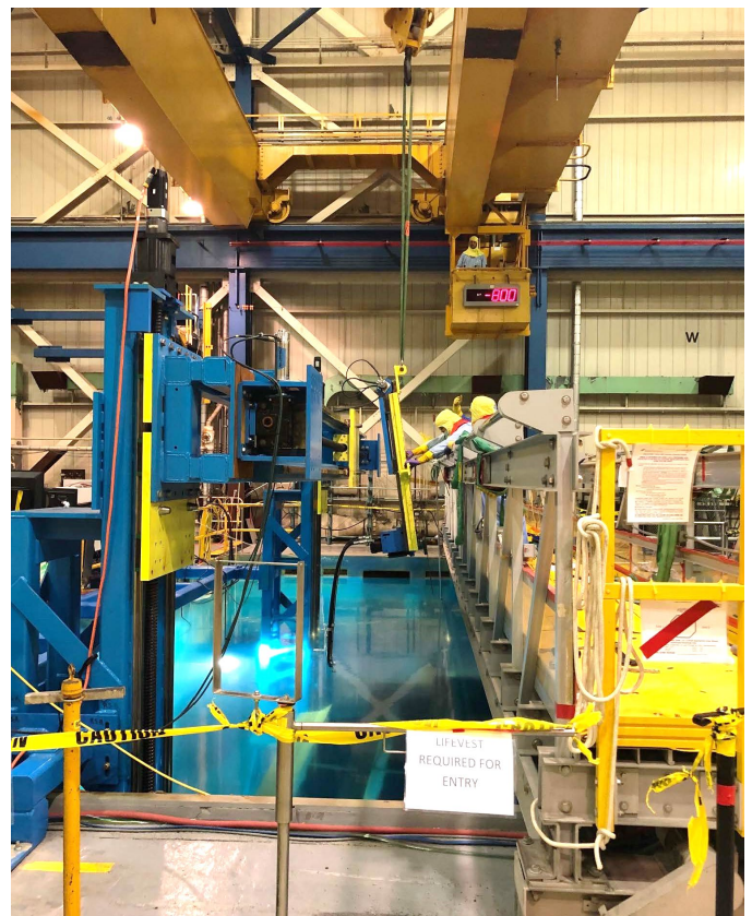
Workers at Oyster Creek Using a Tool Attached to an Overhead Crane to Segment the Steam Dryer, Currently Under Water
