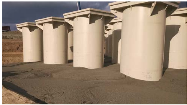
Figure 3: CLSM Pour at the Approximate Halfway Point on the HI-STORM UMAX Cavities
