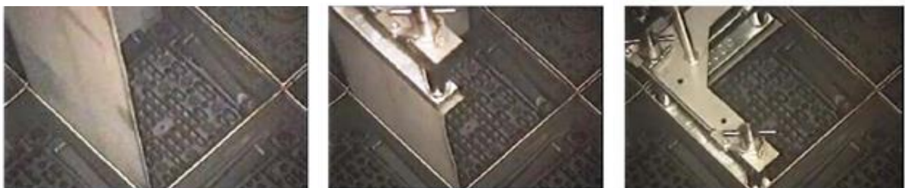
Holtec's DREAM C1 Insert Installation Evolution at FPL's Turkey Point Nuclear Power Plant
