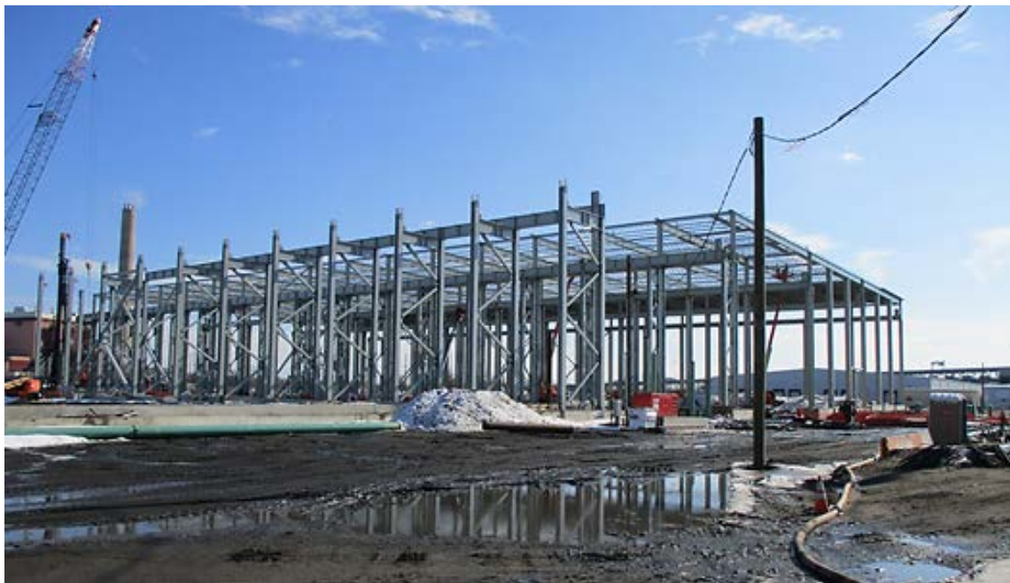
Erection of Steel Girders and Beams for the Heavy Manufacturing Facility (Photo taken February, 2016)
