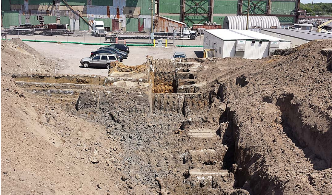
Dilapidated 19th Century Buildings Cleared and Land De-Grubbed for the Engineering Office (Photo taken July, 2015)
