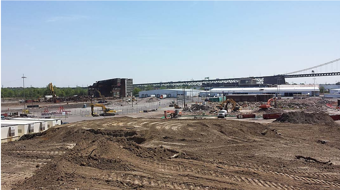
Clearing for the Approx. 2,000 Piles to Support the Heavy Manufacturing Facility (Photo taken July, 2015)
