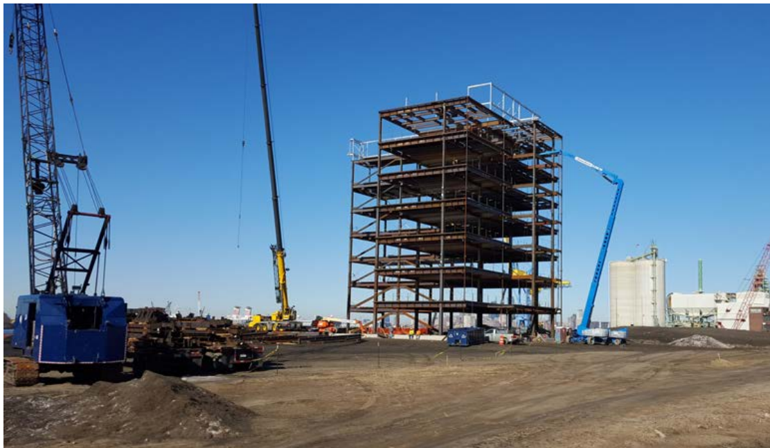
Erection of Steel Support Structures for the Seven-Story Engineering Office (Photo taken February, 2016)
