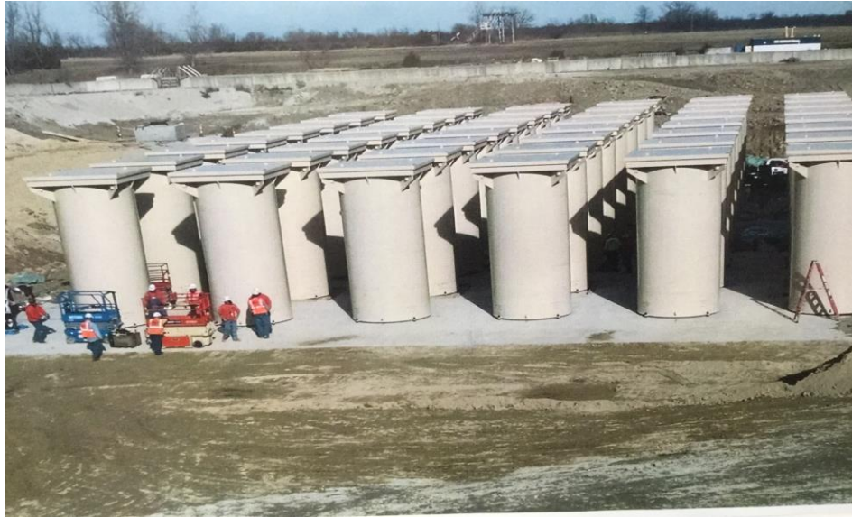
Support Pad complete with 48 CECs set and ready for grouting in November, 2014
