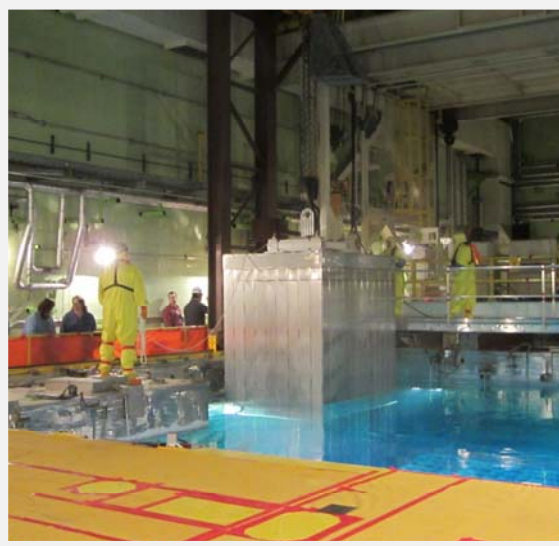
New High Density Rack A1 Being Installed
